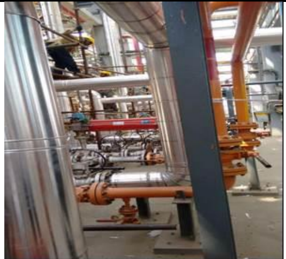
Hot & cold insulation
