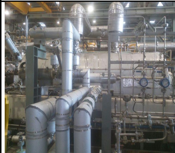
Cold Pipe Insulation
